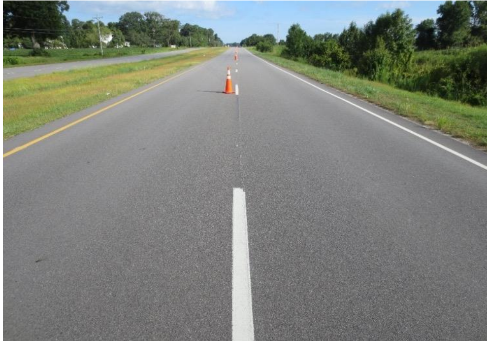
Figure 16. MW RAS WMA (left) and PC RAS WMA (right) at 14-Month Inspection
